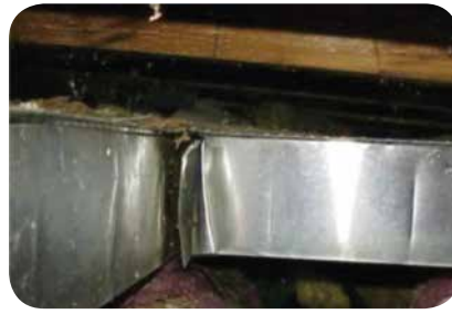
Leaky trunk line to supply duct connection.
