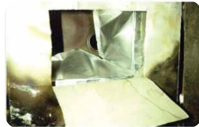
Opened trunk line showing furnace connection.
