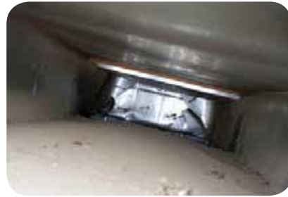
End of trunk line showing unsealed joints
