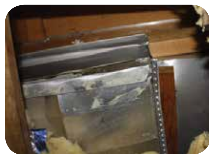
End of trunk line showing unsealed joints
