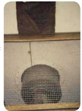
Gap around flue.
