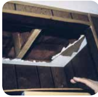
Large hole in ceiling.
